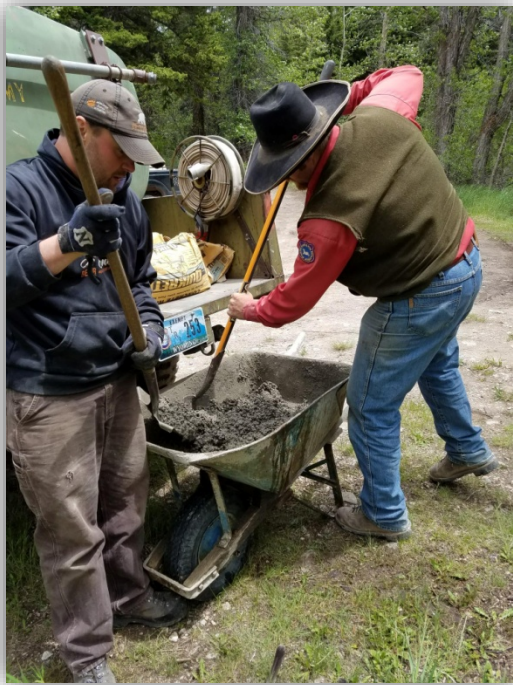
Joe Kondelis from Western Bear Foundation and Miles Proctor from WGFD Habitat and Access mix cement to place a bear box.
